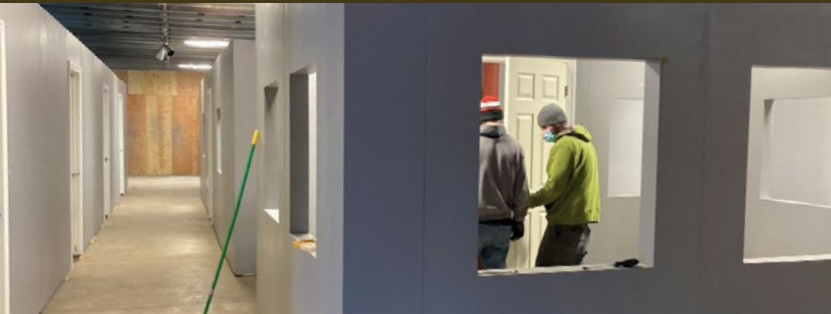
Installing a new Target Identification Training Center for the U.S. Air Force.
